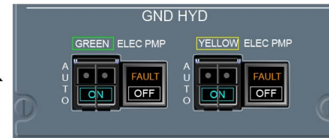
GROUND HYDRAULIC PANEL
