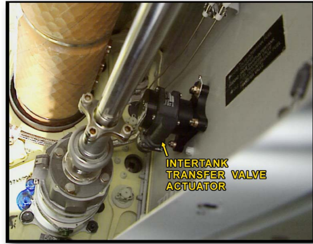
Insulated hot air duct and Valve actuator located outside of the tank
